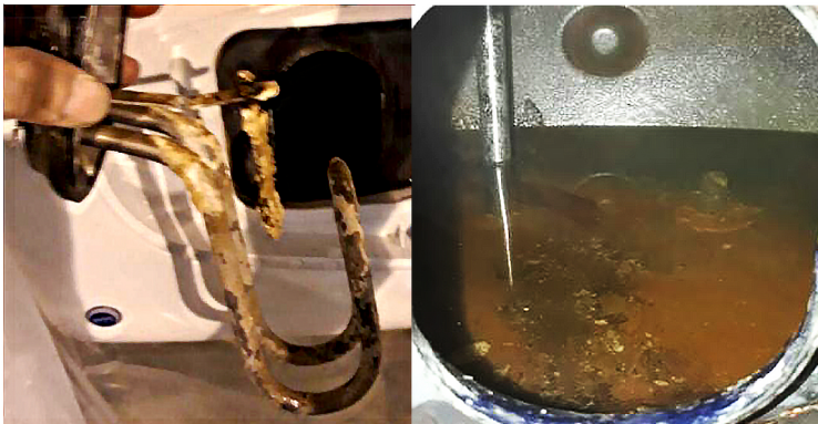
Pictures 5 & 6. 3 weeks after Vulcan installation, initial scale has been eliminated.
