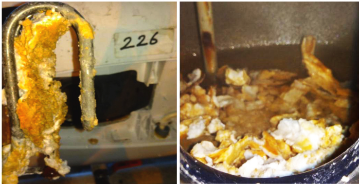
Pictures 2 & 3. Scale previously coating the heating element and reservoir sump. (Picture taken from one of the rooms at IBMA hotel)
